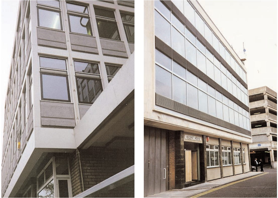
Figure 7 External views of the two multi-storey office buildings showing detail of trickle ventilator installation.
