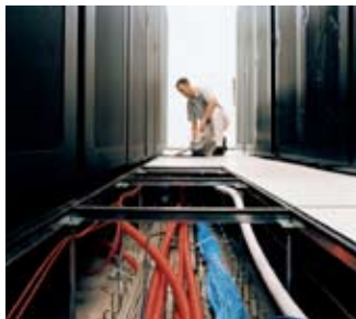
Fig. 79 raised access flooring
