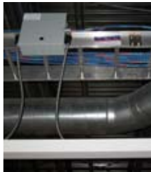
Fig. 50 electrical and telecom raceways
