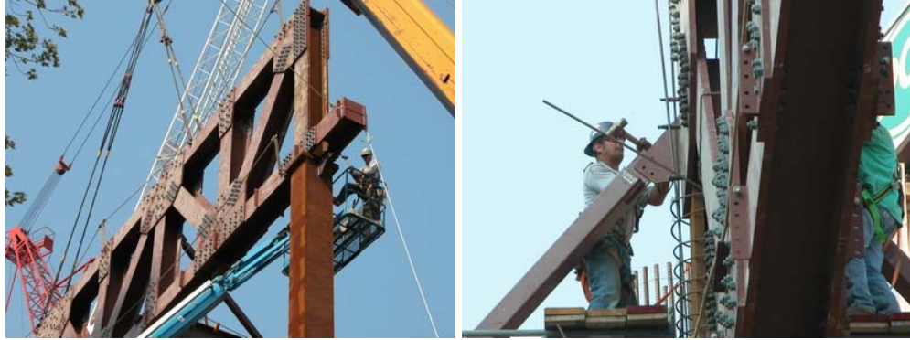
Figures 12 and 13: Leslie Dan School of Pharmacy, University of Toronto, Norman Foster – erection of a 50 tonne steel truss at the fifth floor level.
