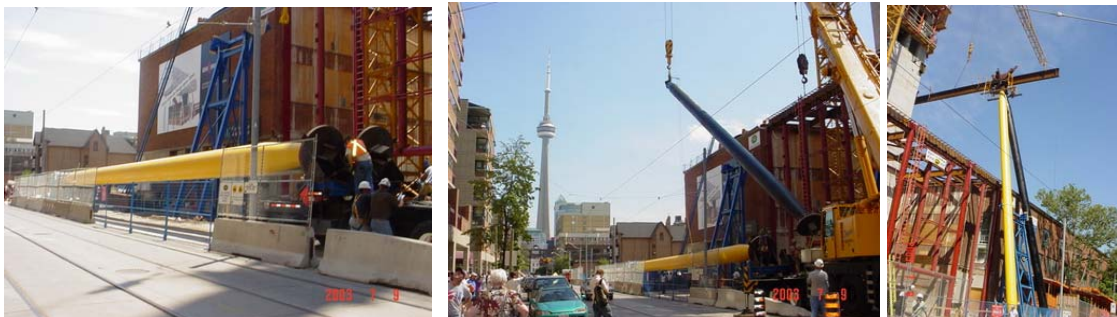
Figures 14, 15 and 16: Erection sequence for HSS legs on OCAD project. Photos: PCL Construction.
