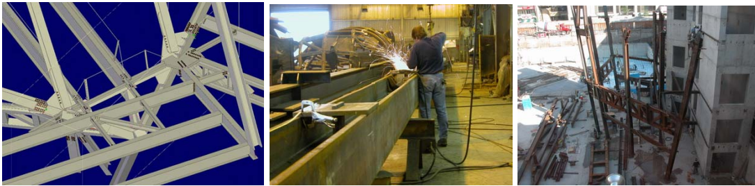
Figures 25, 26 and 27: ROM Addition, Daniel Libeskind: X-Steel joint detail, shop fabrication at Walters Inc., Hamilton, Ontario, erection (project under construction as of September 2004) 7
