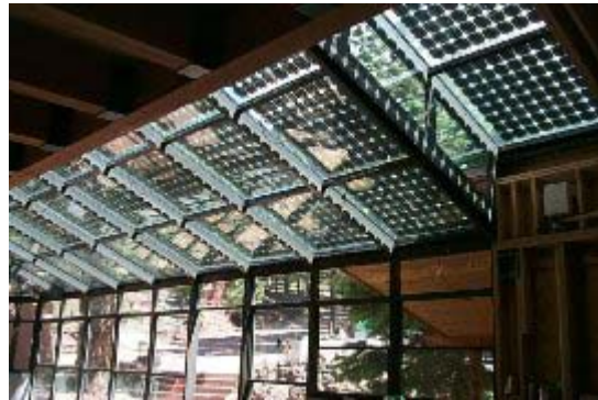
Figure 6 Glass Integrated Photovoltaic (GIPV) provides shade for skylights.
