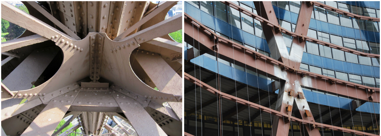
Figure 1. The Eiffel Tower, 1889, was fabricated from members that were built up from plates and angles. The Bow Encana Tower in Calgary, Foster + Partners, 2011, used a wider variety of members from which to fabricate the large custom steel sections of its double glazed façade.
