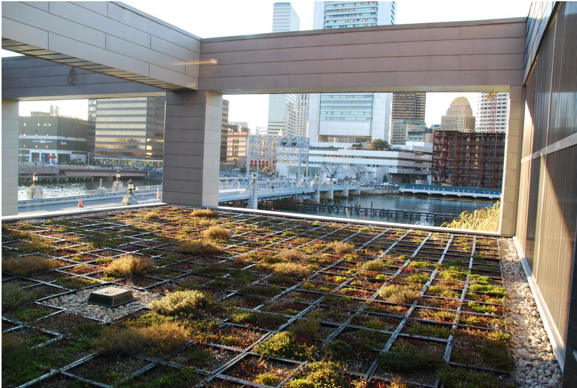
Boston Children's Museum: green roof panels/squares
