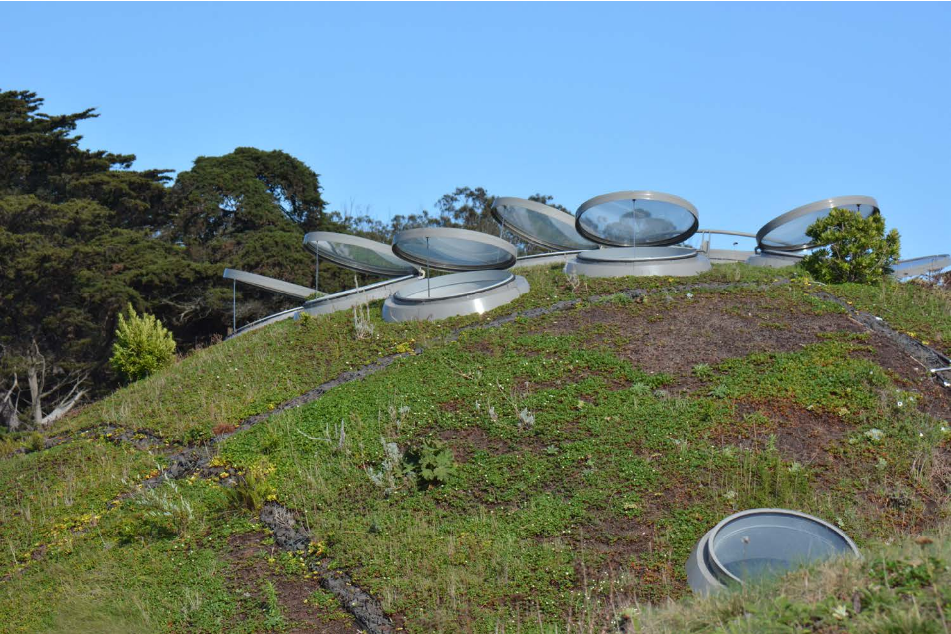
Operable skylights to vent heat from interior
