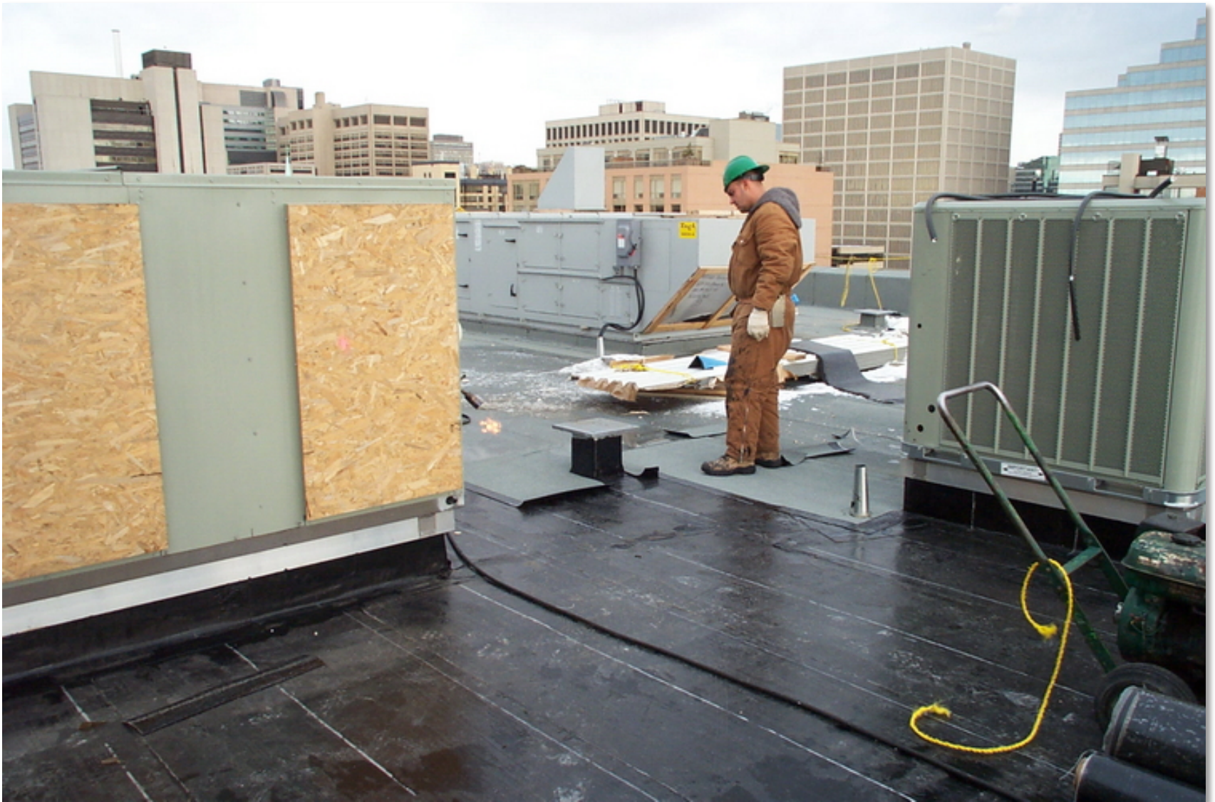
This is the roofing membrane being installed on the top of the new OCAD addition.
