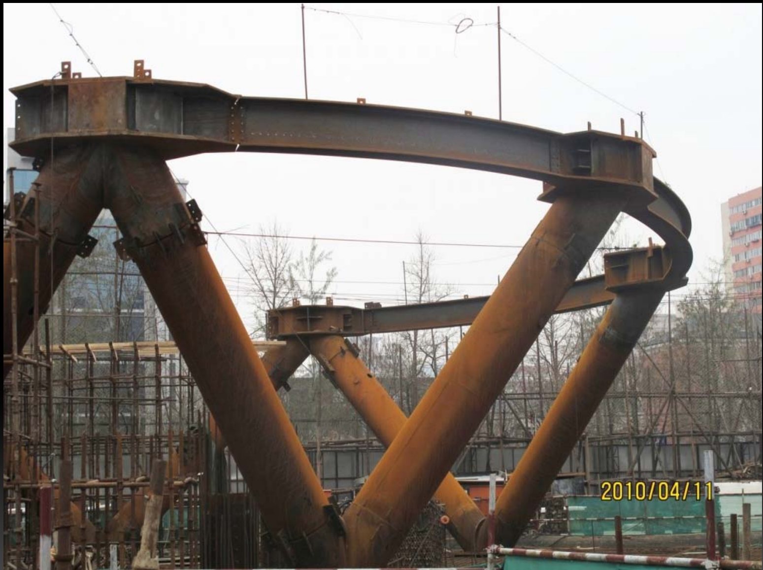
Ground floor support steel goes in. Use of tubes and welded connections.
