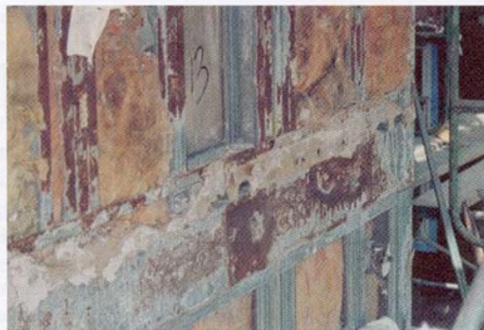
Figure 1: View of severely corroded hot-dip galvanized structural members due to poulitice corrosion from wet building sheathing. Metal loss exceeded 20% of original thickness.
