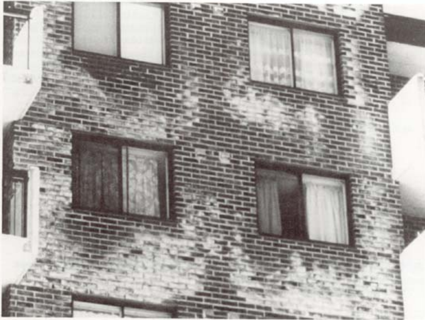
Fig. 16 An example of extensive wetness and efflorescence
