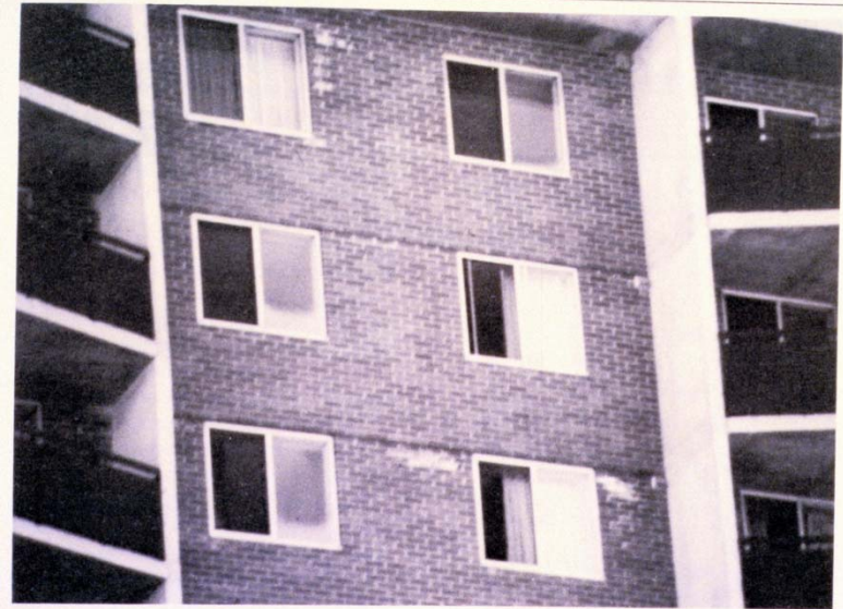
Fig. 15 Example of air leakage on the side of a building
